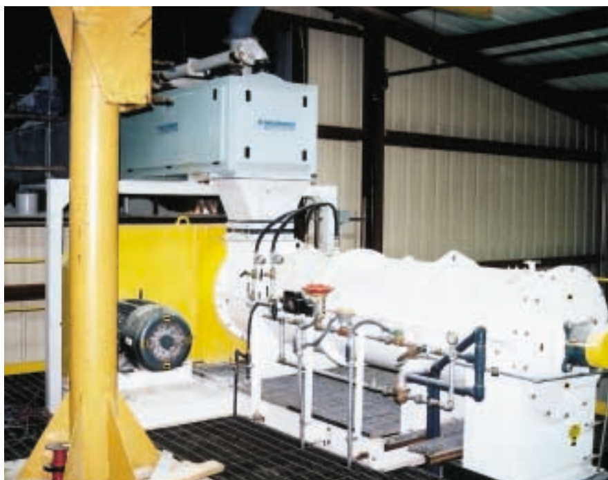
The agglomeration process begins in the continuous pin mixer as the binder solution mists over the powdered limestone.
