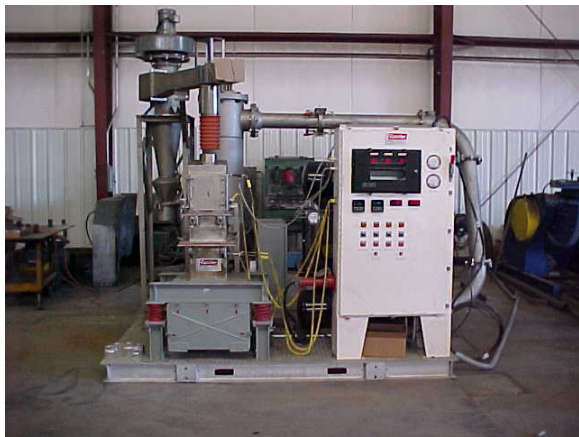
Photo 5 - Batch Fluid Bed Dryer
